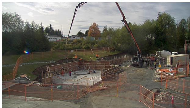
Construction is underway for the mobile CT pad at the Port Hardy Hospital
